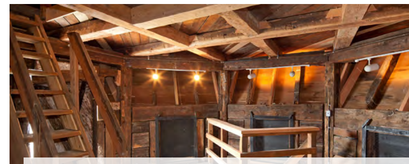
The Bastion | Structural and Building Envelope Restoration | Nanaimo, BC AWARD | 2011 Heritage Conservation Outstanding Achievement Award | Heritage BC AWARD | 2011 Heritage Building Rehabilitation Award | City of Nanaimo
