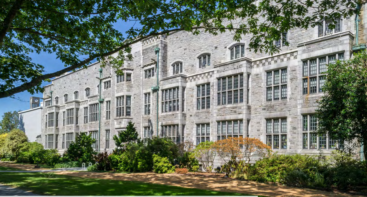
University of British Columbia Chemistry Centre | Façade and Window Conservation | Vancouver, BC
