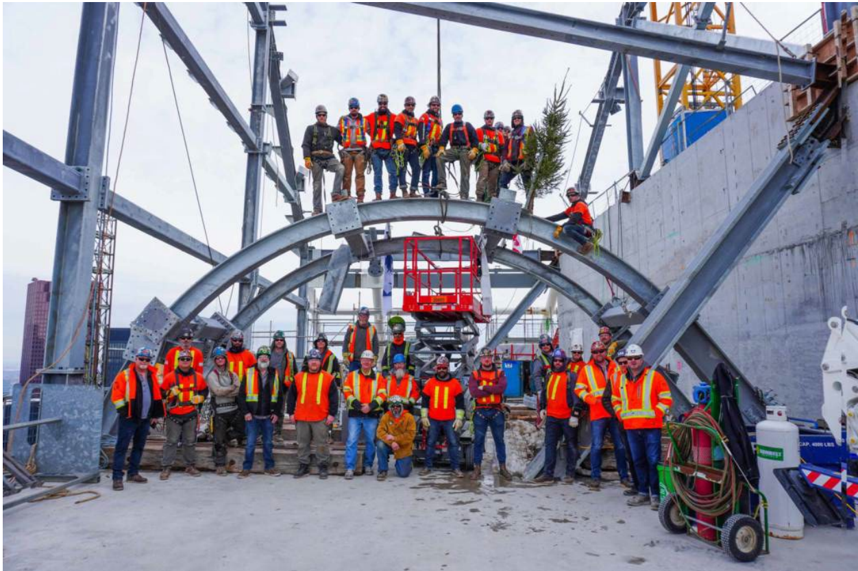
Image 3 of 4 - A view of the construction team perched on the top of the steel structure.
