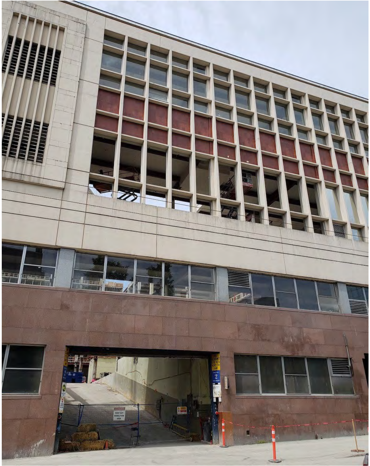
Construction progress on the Canada Post redevelopment in downtown Vancouver on June 10, 2019. (Kenneth Chan/Daily Hive)
