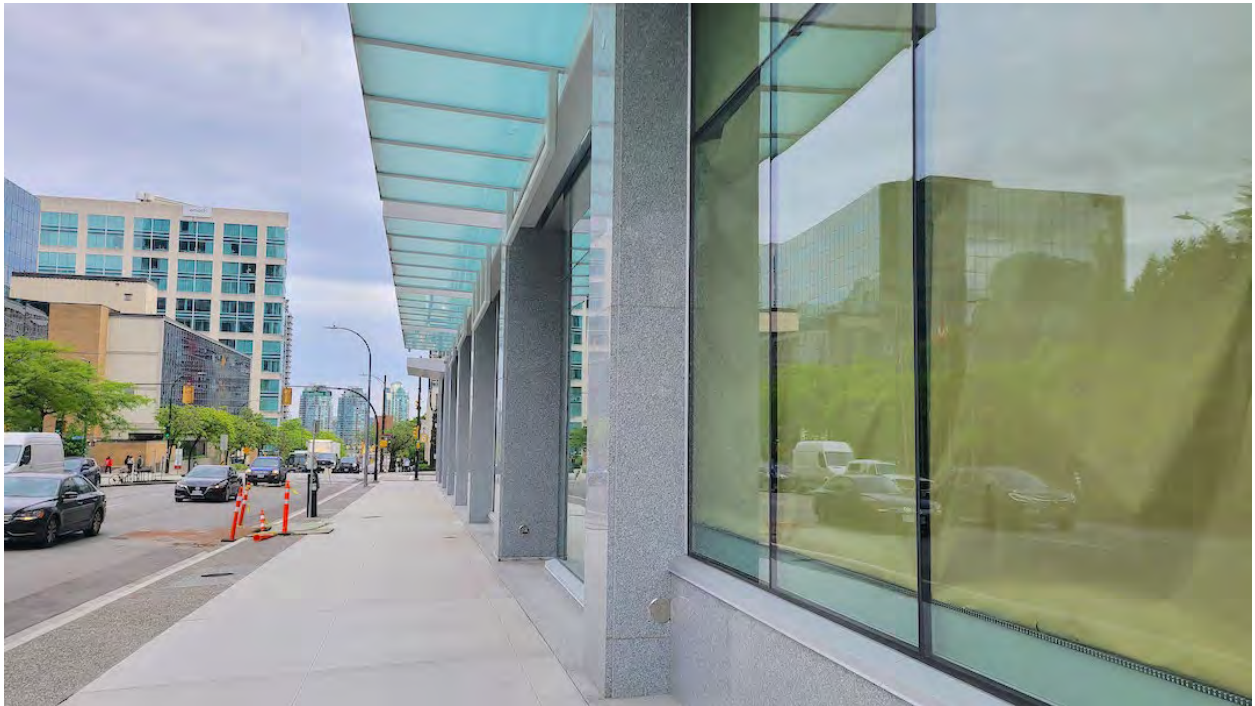
Exterior of The Post; Construction progress as of May 23, 2023. (Kenneth Chan/Daily Hive)
