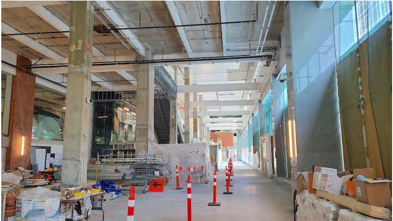
Future retail concourse of The Post; Construction progress as of May 23, 2023. (Kenneth Chan/Daily Hive)
