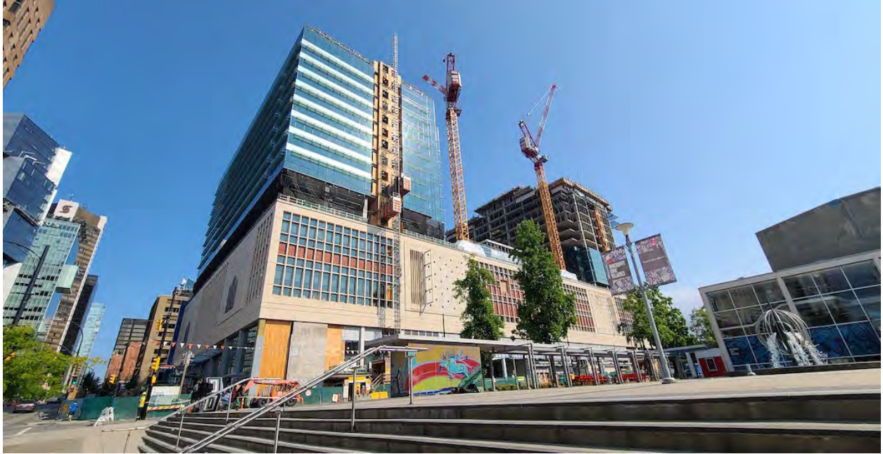
Construction progress of The Post in downtown Vancouver, as of June 29, 2021. (Kenneth Chan/Daily Hive)
