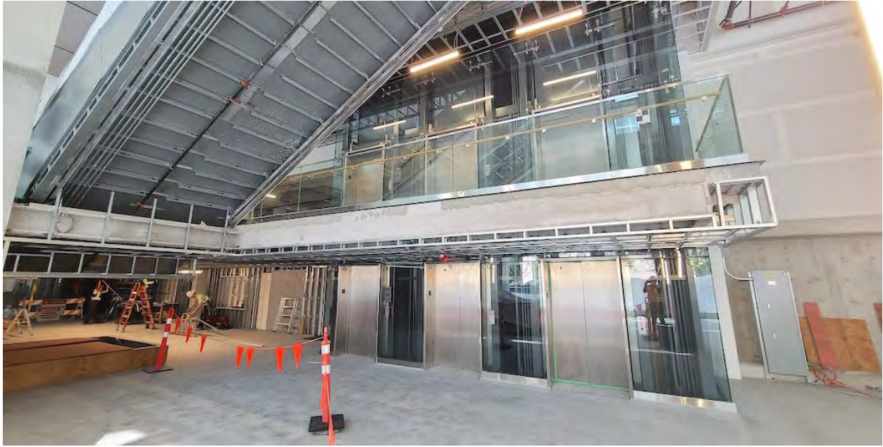
Future retail concourse of The Post; Construction progress as of May 23, 2023. (Kenneth Chan/Daily Hive)
