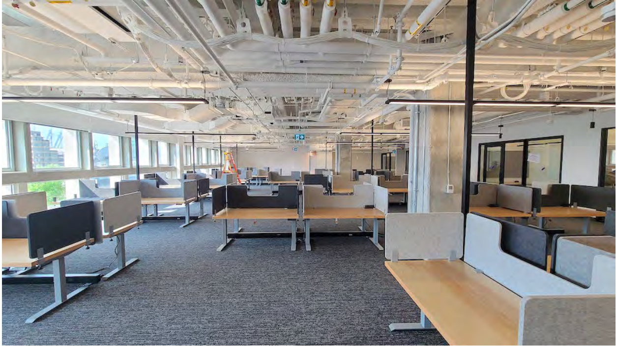
Amazon office space being furnished inside The Post's South Tower; Construction progress as of May 23, 2023. (Kenneth Chan/Daily Hive)
