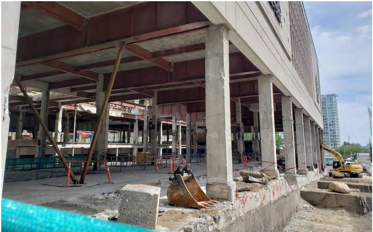
Construction progress on the Canada Post redevelopment in downtown Vancouver on June 10, 2019. (Kenneth Chan/Daily Hive)
