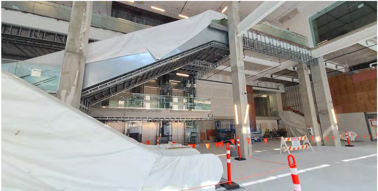
Future retail concourse of The Post; Construction progress as of May 23, 2023. (Kenneth Chan/Daily Hive)
