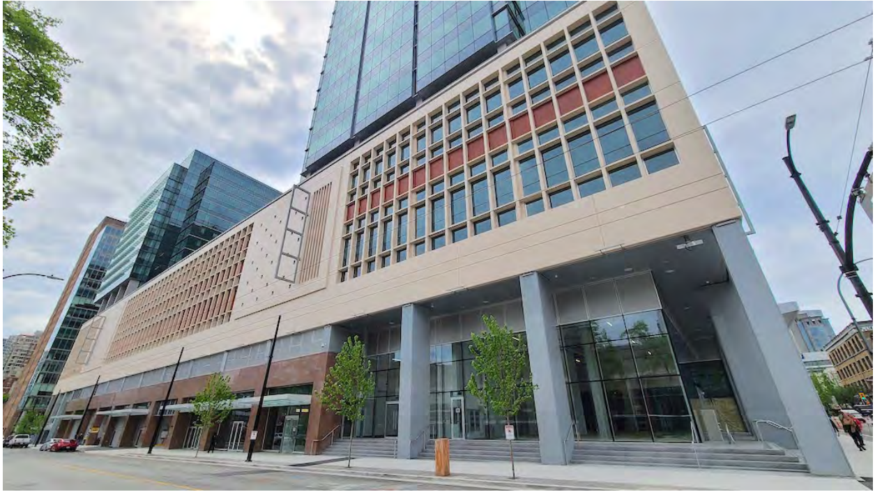
Exterior of The Post; Construction progress as of May 23, 2023. (Kenneth Chan/Daily Hive)
