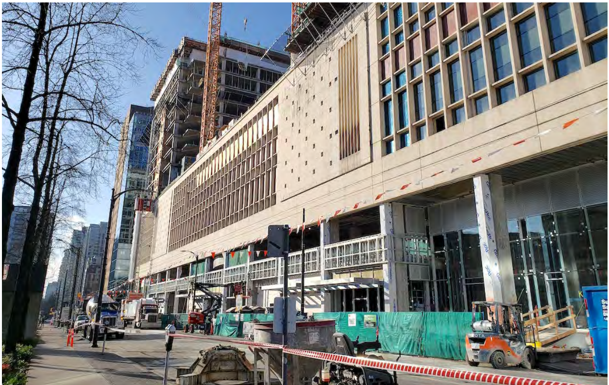
Construction progress of Amazon's new Vancouver offices at The Post, as of January 15, 2021. (Kenneth Chan/Daily Hive)
