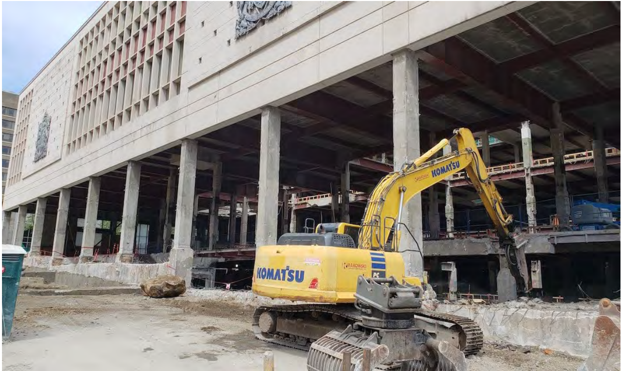
Construction progress on the Canada Post redevelopment in downtown Vancouver on June 10, 2019. (Kenneth Chan/Daily Hive)
