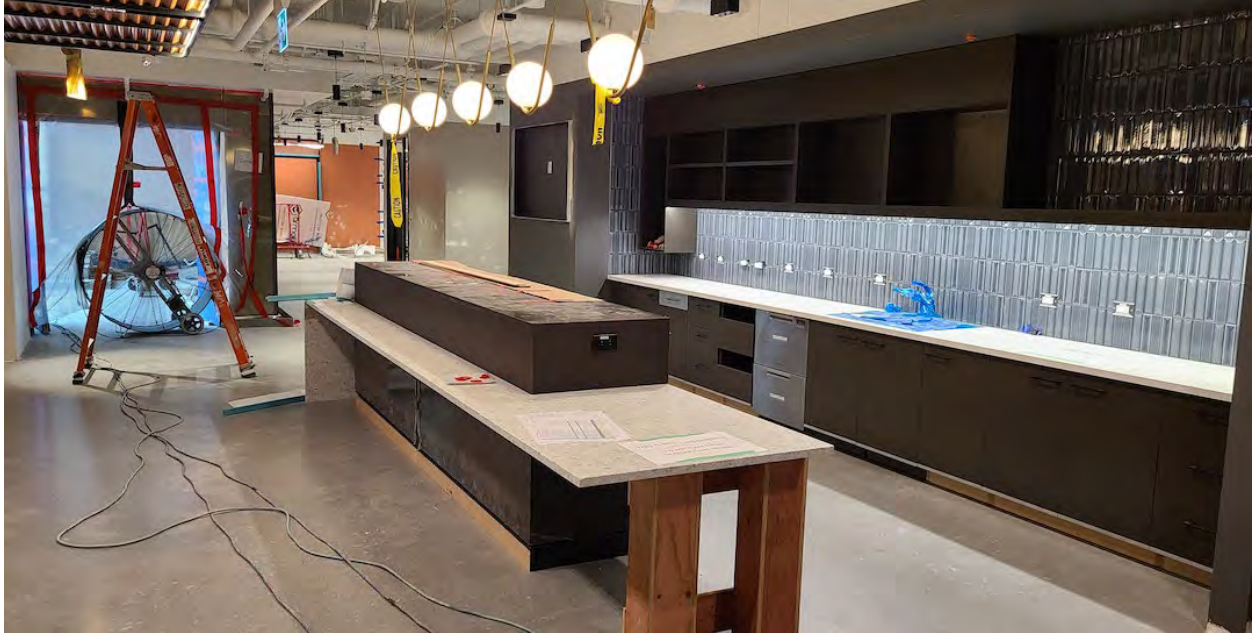
Amazon office space being furnished inside The Post's South Tower; Construction progress as of May 23, 2023. (Kenneth Chan/Daily Hive)
