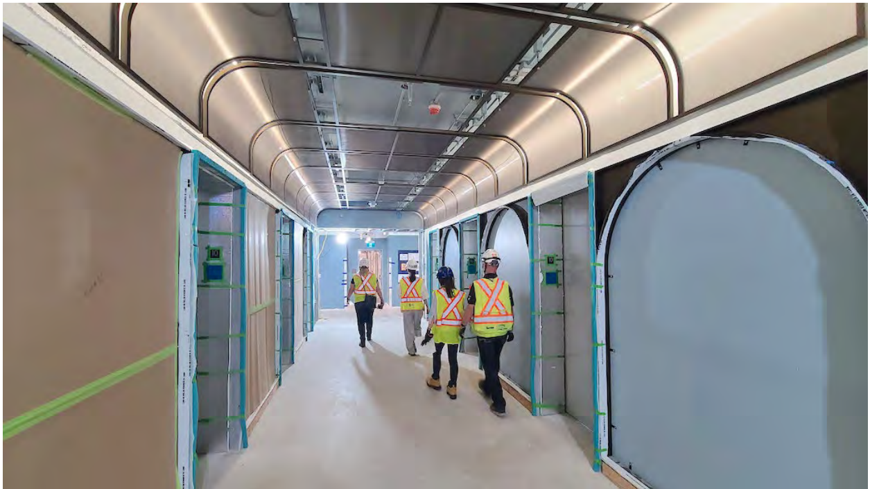
Amazon office space being furnished inside The Post's South Tower; Construction progress as of May 23, 2023. (Kenneth Chan/Daily Hive)
