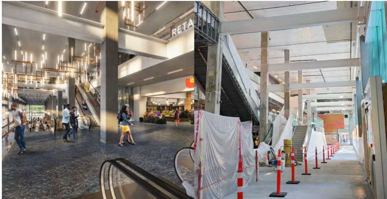
Artistic rendering of the retail concourse of The Post (left) and construction progress as of May 18, 2023 (right). (Kenneth Chan/Daily Hive)
