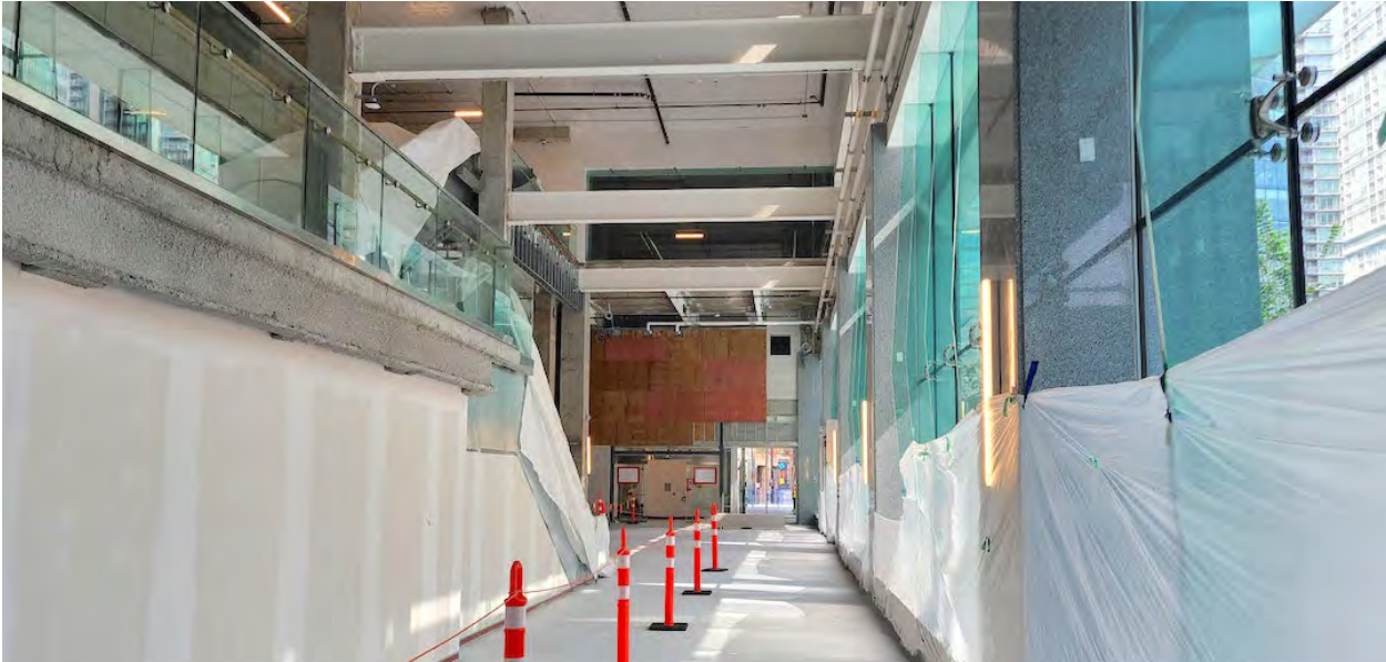
Future retail concourse of The Post; Construction progress as of May 23, 2023. (Kenneth Chan/Daily Hive)
