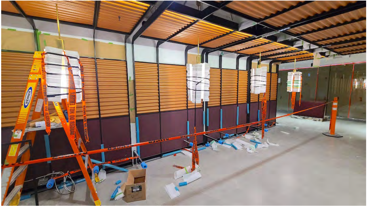
Amazon office space being furnished inside The Post's South Tower; Construction progress as of May 23, 2023. (Kenneth Chan/Daily Hive)
