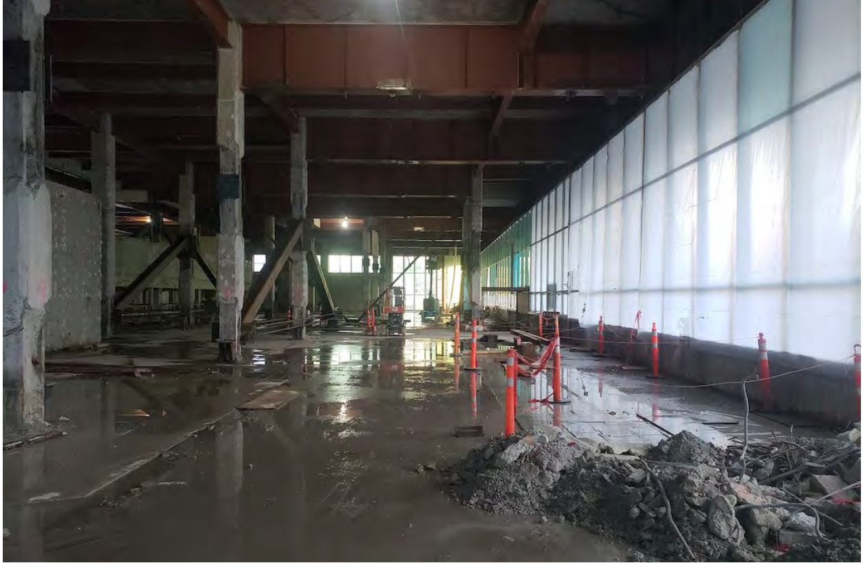
Construction progress on the Canada Post redevelopment in downtown Vancouver on March 26, 2019. (Kenneth Chan/Daily Hive)
