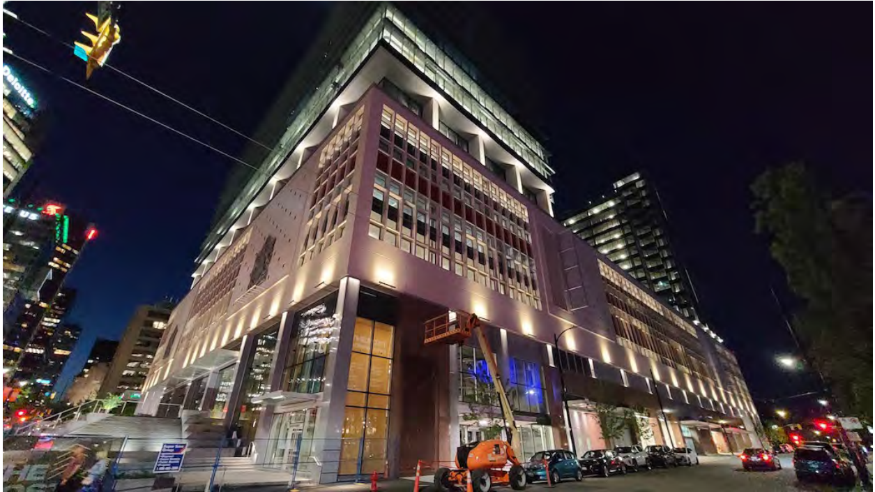
Exterior of The Post; Construction progress as of May 23, 2023. (Kenneth Chan/Daily Hive)
