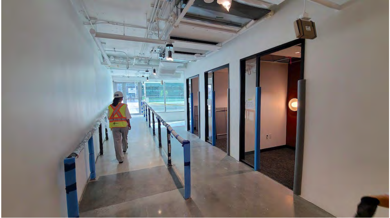
Amazon office space being furnished inside The Post's South Tower; Construction progress as of May 23, 2023. (Kenneth Chan/Daily Hive)
