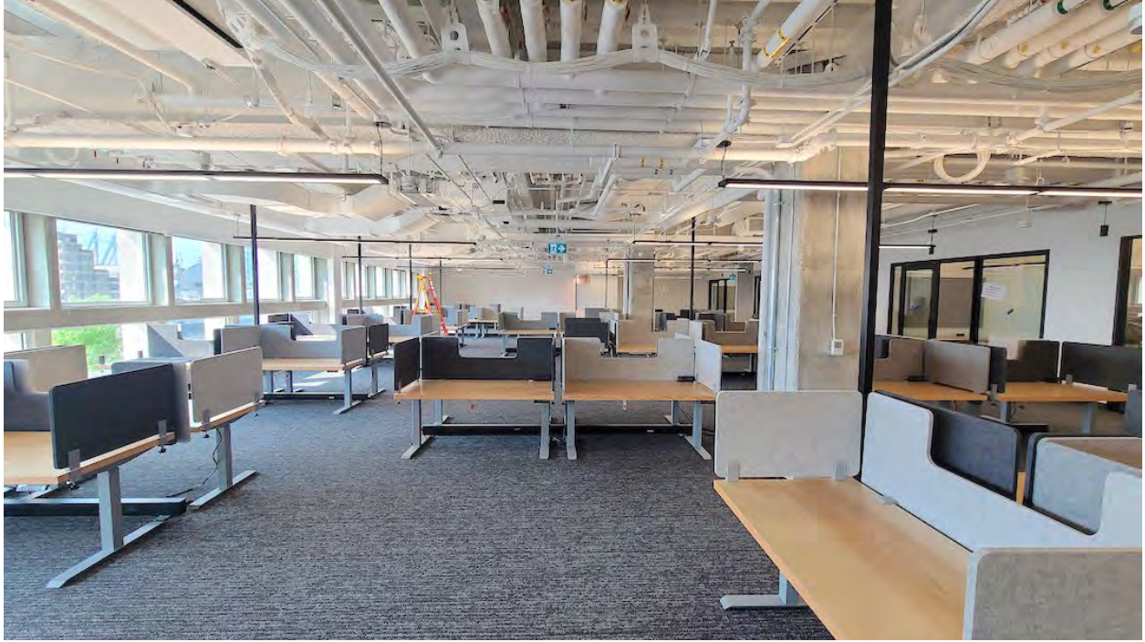
Amazon office space being furnished inside The Post's South Tower; Construction progress as of May 23, 2023. (Kenneth Chan/Daily Hive)
