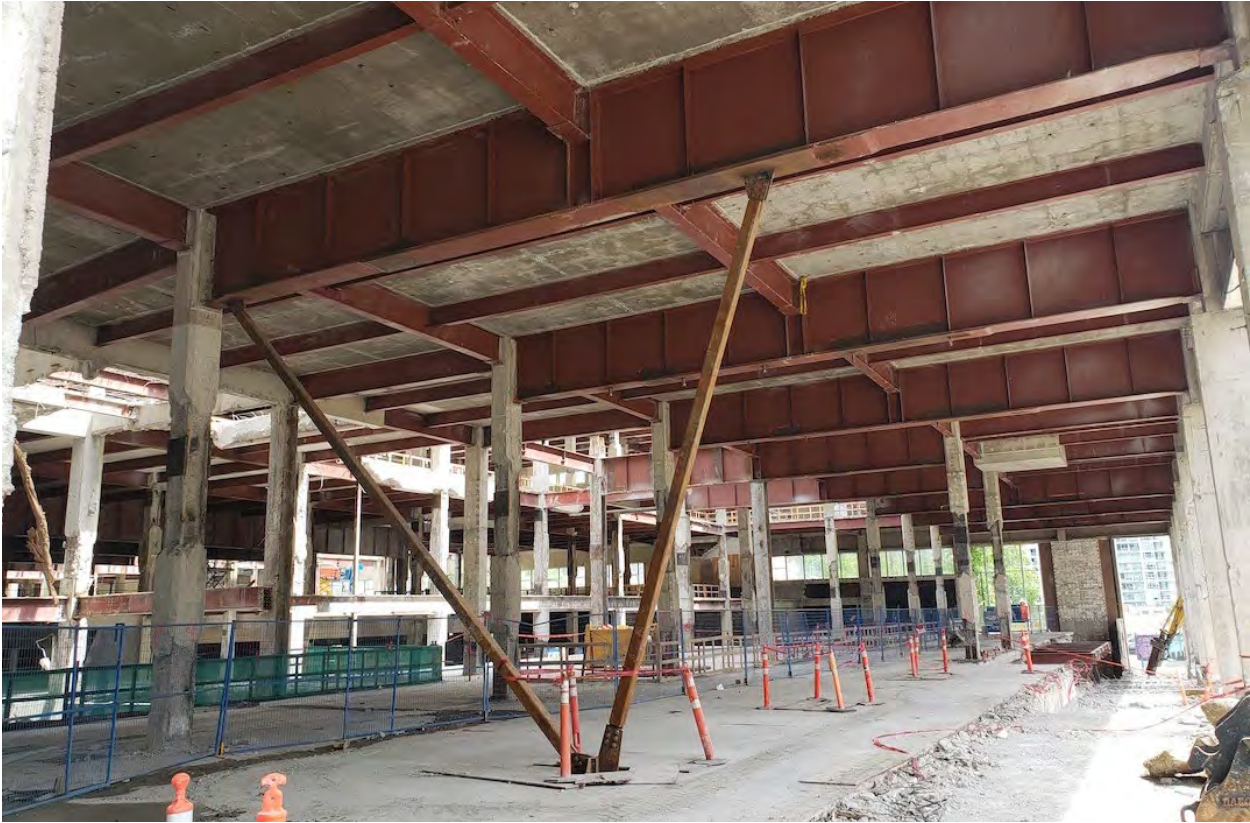
Construction progress on the Canada Post redevelopment in downtown Vancouver on June 10, 2019. (Kenneth Chan/Daily Hive)
